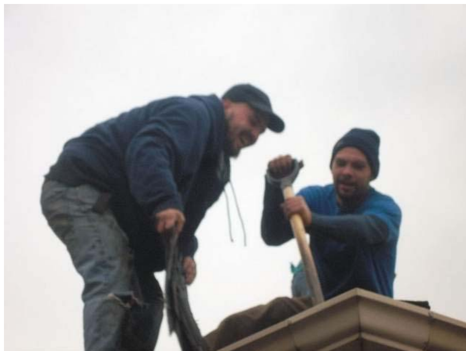
Mike Sanchez and Dwight Warlick of Northwest Construction dig into Elaine Collings's roof.
